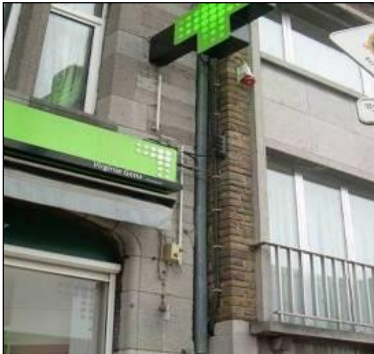
Multiport on facade
