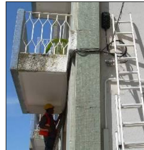
FlexNAP tap hidden under balcony
