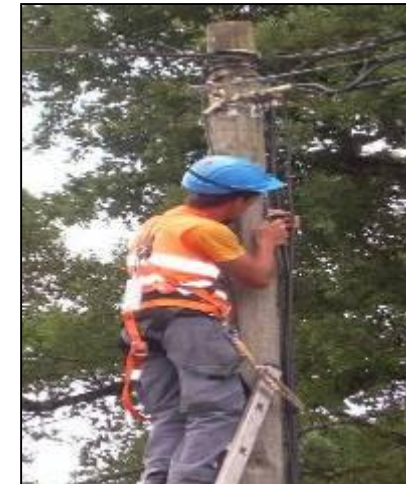
Connecting pre-connectorized drop- cable
